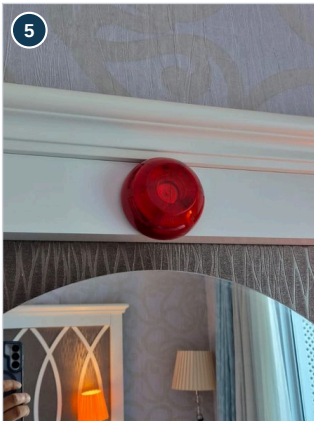
Fire alarm warning device in the room
