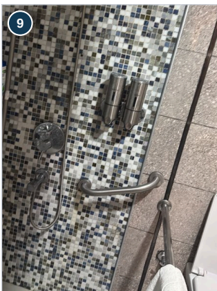
Horizontal grab bar and soap dispensers on the shower wall
